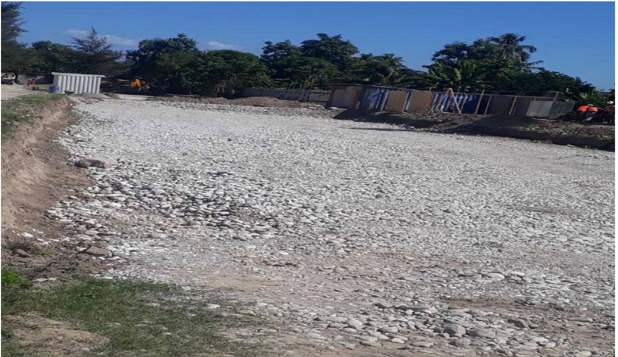
Second layer of backfill in classrooms awaiting compaction test by the building laboratory (LNBTP)
