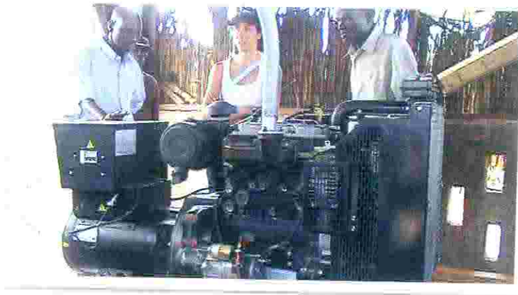
Fig 7: the 27 KVA perkins generator handed over to Whelmer water supply
